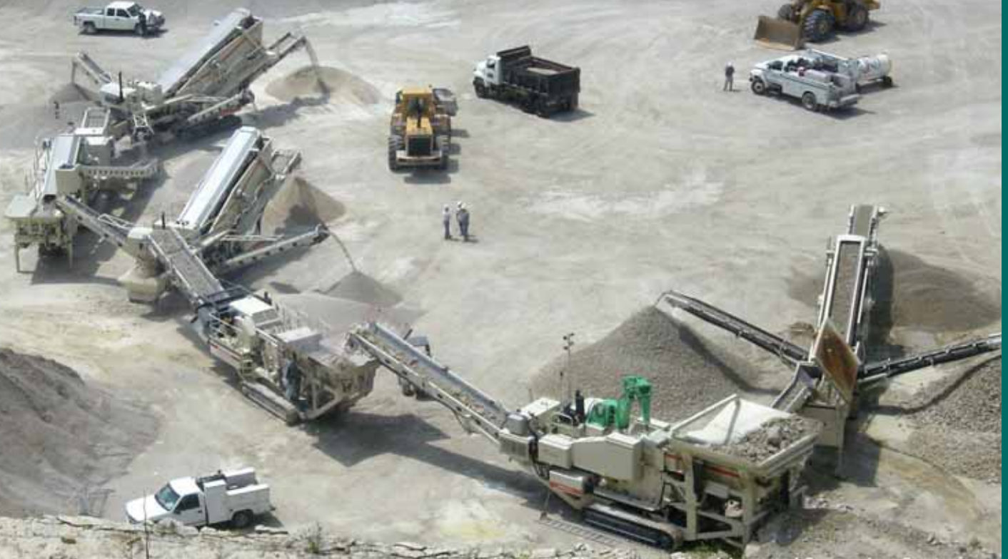
Lokotrack Five-Stage Crushing and Screening System at Capital Quarries site in Owensville, MO
